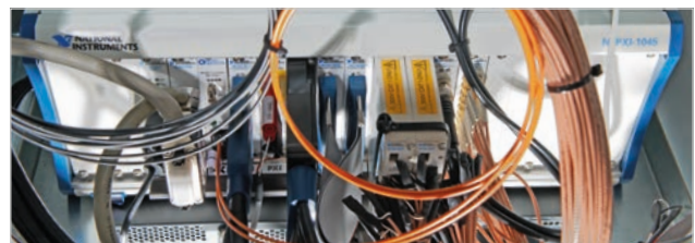
Internal wiring on the PXI core system
